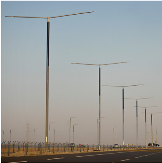
Ghayathi Highway, Abu Dhabi, U.A.E. Worldwide first 100 % solar and 100% off-grid highway lighting
