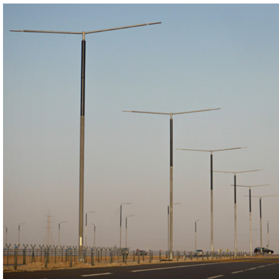
Gayathi Highway, Abu Dhabi, U.A.E. Worldwide first 100 % solar and 100% off-grid highway lighting
